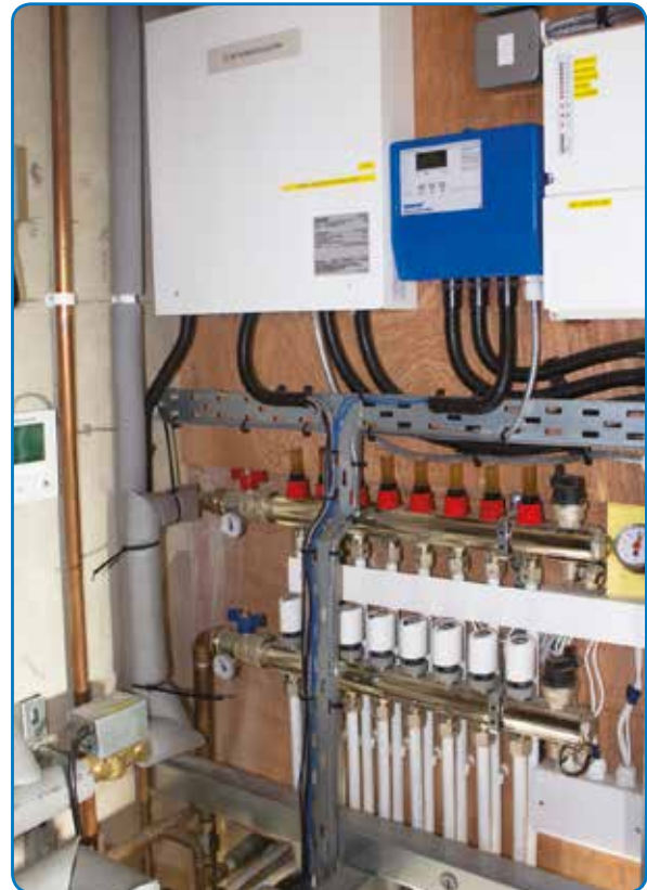
UFH manifold in the ground floor plant room showing the air source heat pump control unit and a T2 Topway manifold. In addition an Emmeti EWC1 wiring centre provides central electrical control to all system components including room thermostats, electrothermic heads and the heat source.
