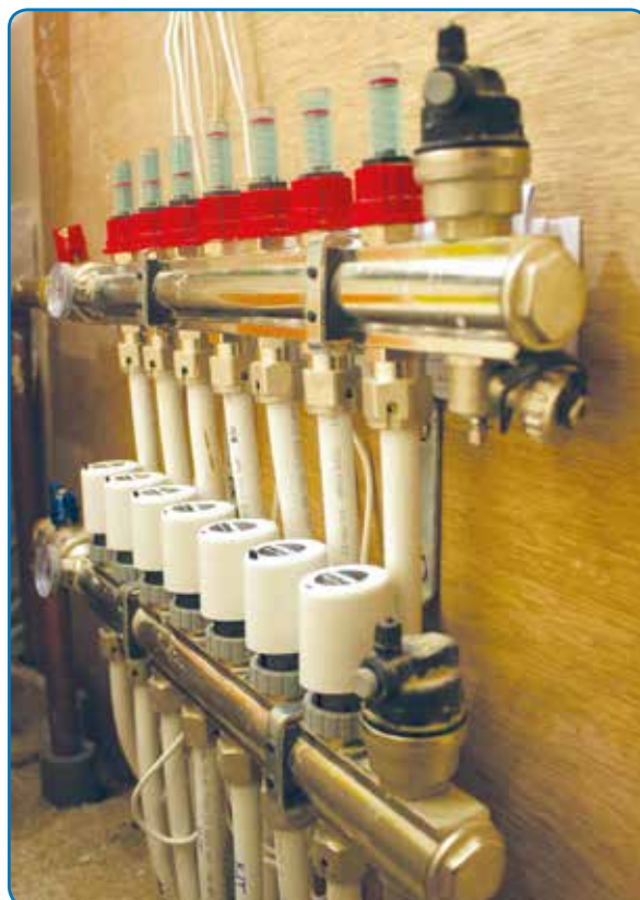
The Ground floor uses an Emmeti T2 Topway heating manifold (7 port) to supply seven individual UFH loops. The integrated double regulating flowmeters on the top flow rail allow for individual circuit flow control to ensure correct balancing of systems. The integrated electrothermic valves on the lower return rail allow for electrical control of each circuit via electrothermic actuators.
